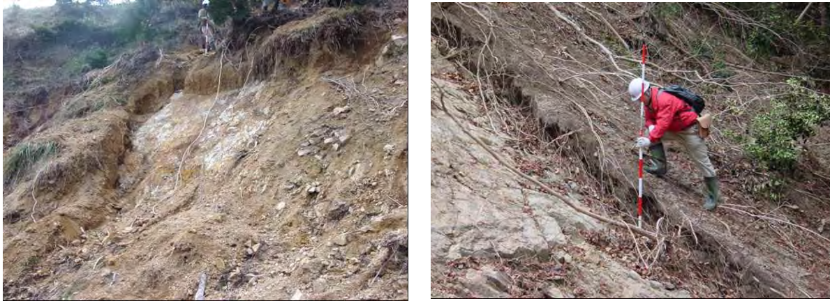
Fig. 5, Translational failure in weathered granite
